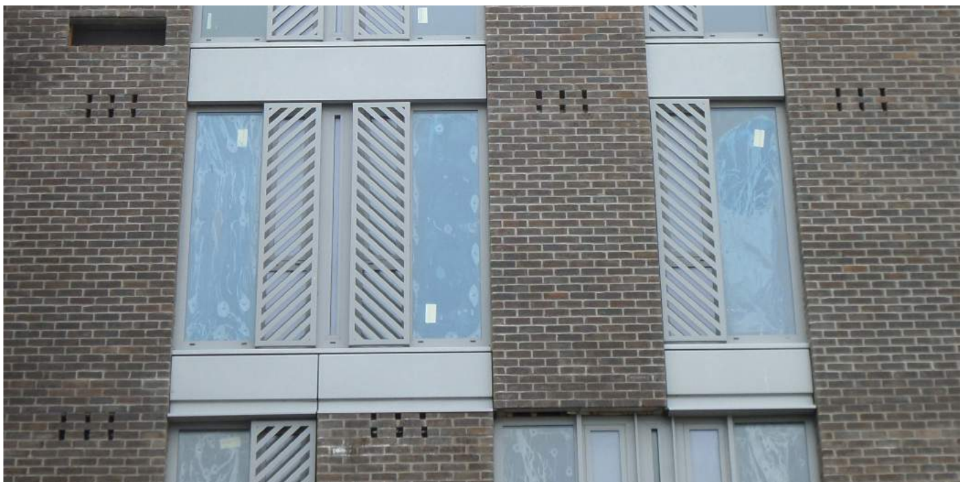
View of ventilation perpendes
